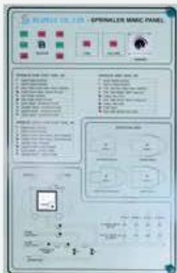
Sprinkler MIMIC Panel
