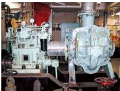
Fire Pump Unit
