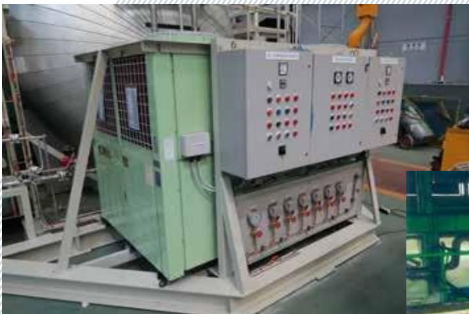
Refrigerating unit & Control Panel
