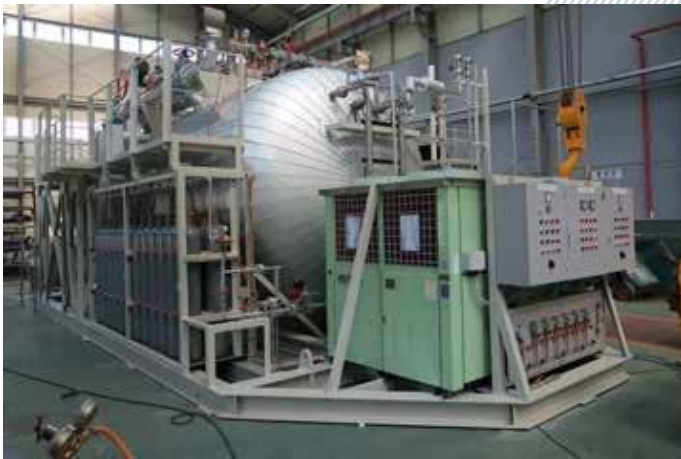
Low Pressure CO 2 Storage Unit
