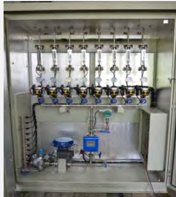
SCR+SNCR系统分配柜 SCR+SNCR system distribution cabinet
