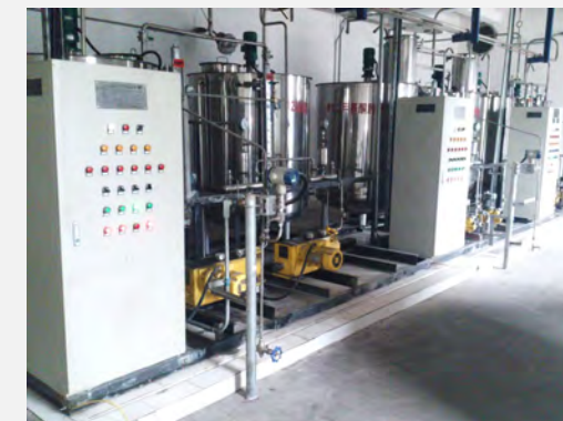
WS2200炉内加药系统 WS2200 Furnace Dosing System
